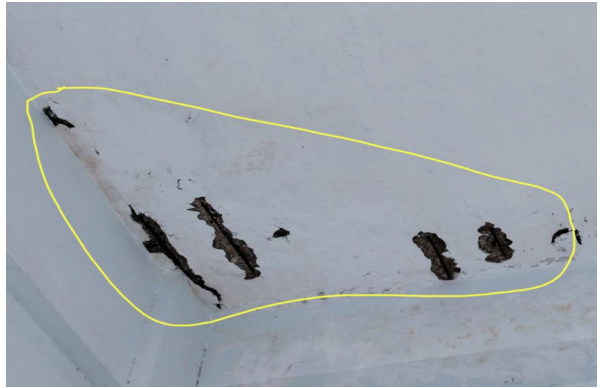
Fig. 4. Rebar Corrosion of Stair Case Roof Slab
