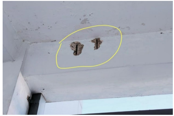
Fig. 3. Concrete Spalling on Roof Beam Second Floor
